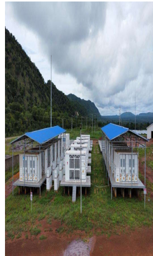
30 MWh BESS to Hybrid Generation
