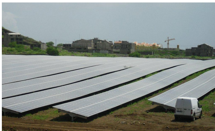
5 MW Grid-Connected PV Station in Praia, Cape Verde: The current largest installation in Sub Sahara Africa
