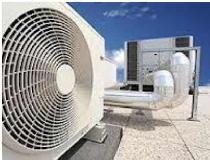
Cooling, ventilation air conditioning
